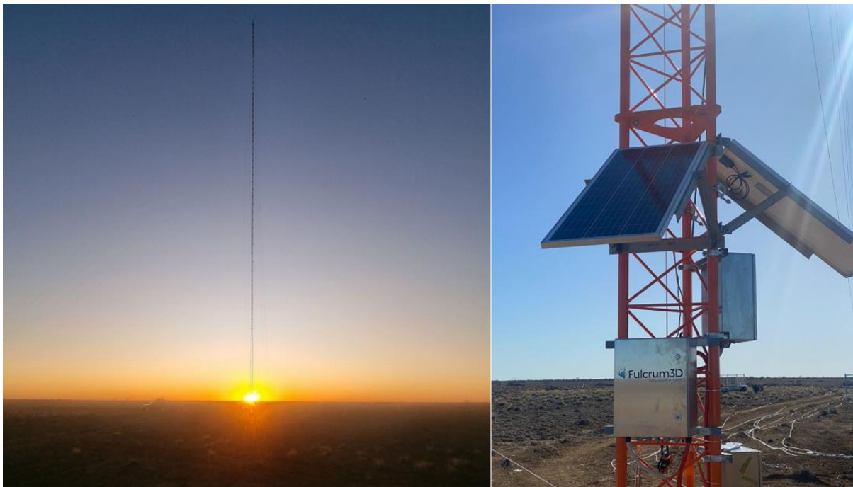
QEM's met mast was commissioned during the September quarter.
